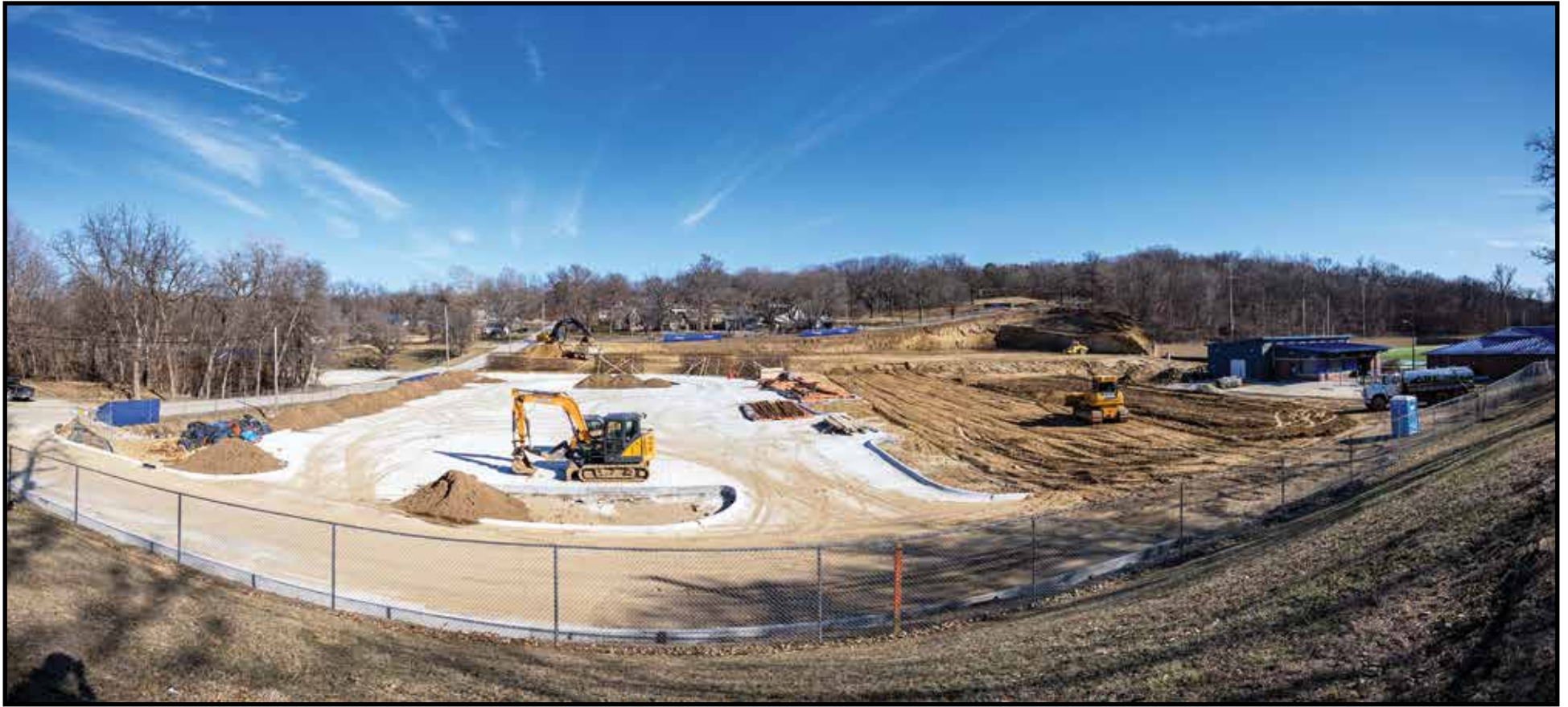
Recreation Dome Construction, February 2024 Aerial Photo by Peru State College Marketing Department and submitted by Ted Harshbarger.
